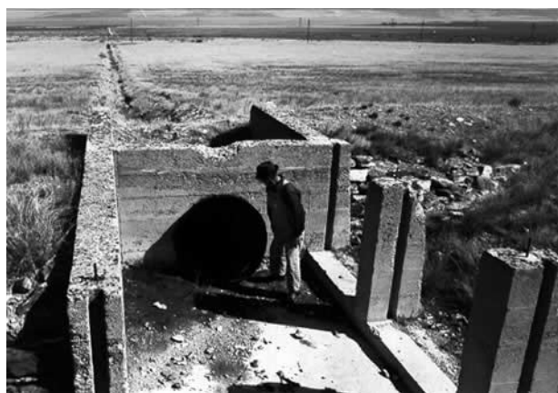
Photograph 2. Alva Moore Jr. inspects remains of bifurcation structure located a mile and a quarter west of the pumping
